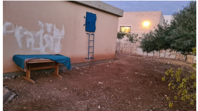
The Youth Center is currently in an old building desperately in need of painting, repairs and a garden
